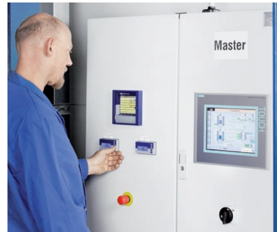
The master control cabinet coordinates the functions of the various plant components.
