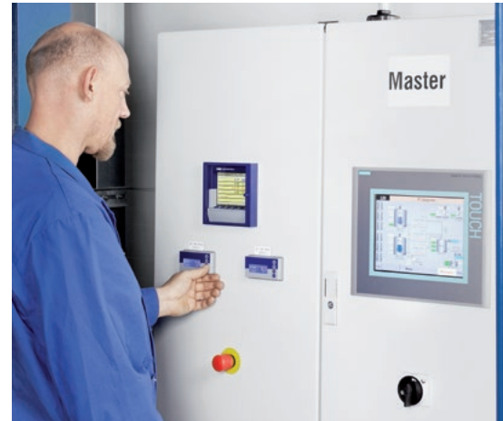
The master control cabinet coordinates the functions of the various plant components.
